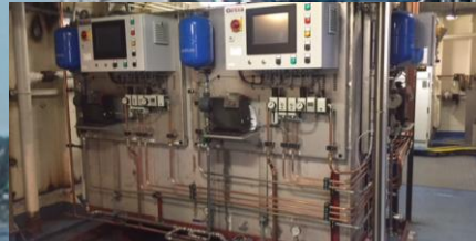
Urea tank with dosing unit and control system
