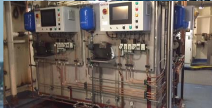
Urea tank with dosing unit and control system
